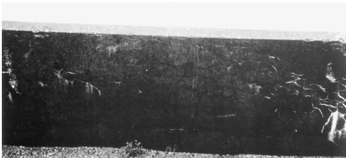
FIG. 3. Panel No. 24-4 (Notice Efflorescence, Pattern Cracking and Change of Color)
