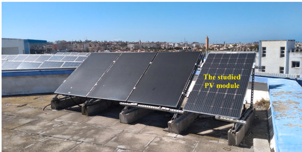
Fig. 4. Real view of the SEAC60T-300 polycrystalline PV panel installed in El Jadida.
