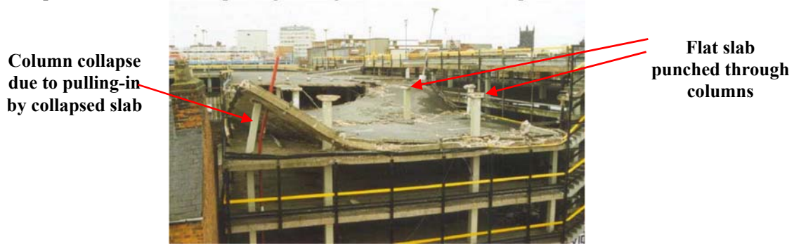
Figure 1. Collapse of large area of flat slab due to punching shear [1]
