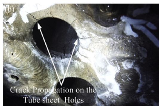
Fig. 19. SCC cracks at tube-to-tubesheet joints [281].
