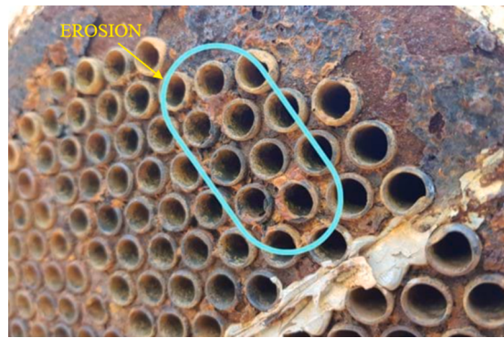
Fig. 7. Erosion at Tube-to-tubesheet [50].
