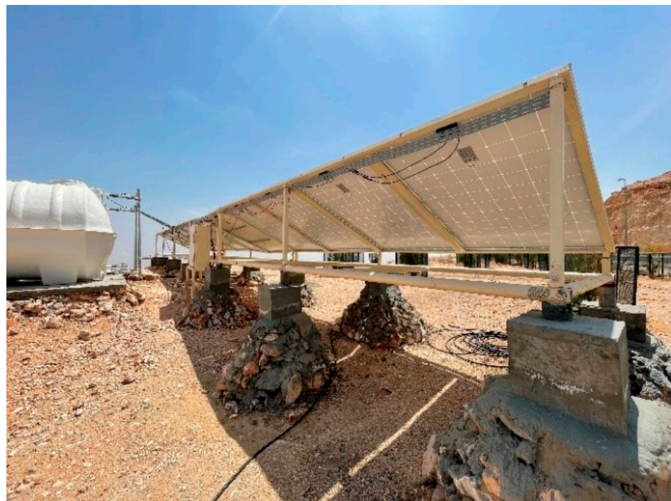
Figure 2. Taken at Hafeet Mountain for the water tanks powered by solar panels.
